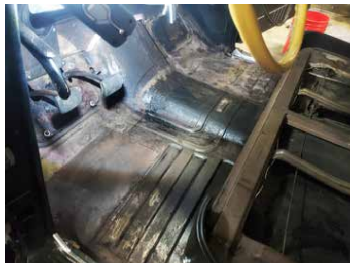
Remove the carpets and any pre-existing insulation so you have clean metal as a base.
