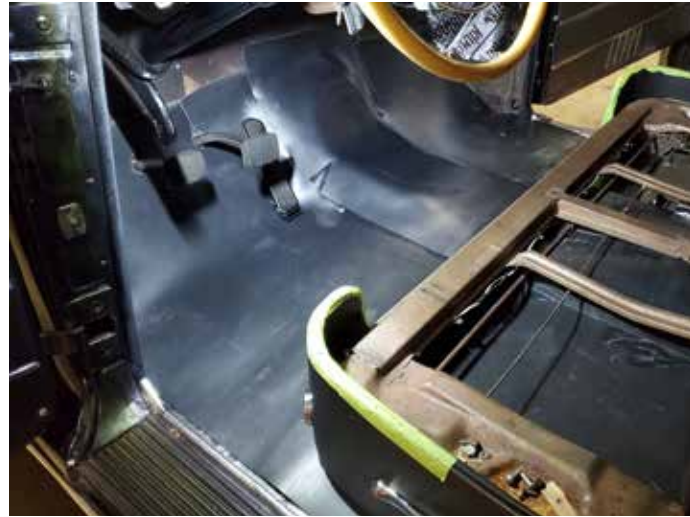
Three pieces of MLV cover front seat area. Note the pie-cuts to help the MLV conform to the transmission tunnel.
