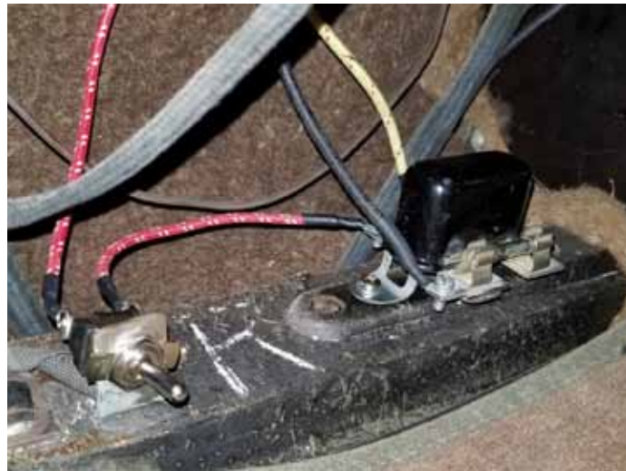
13. I made a bracket for the toggle switch and hid it under the dash where it can be reached easily. Then I installed the relay nearby where it will be safe and dry. Sorry, I don't know what the "R" stands for.
