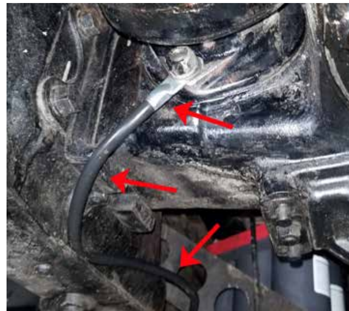
Install another ground cable from the starter to a ground point as close to the battery ground as possible.
