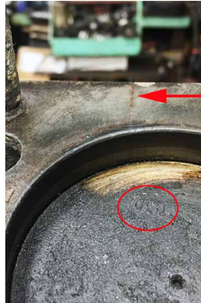
Damage to the Lincoln's block extended to the deck surface (arrow). Note that the block has been sleeved and fitted with .030" oversize pistons (circle). Someone knew about the damage and simply ignored it.
