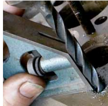
Use a square to keep your drill bit perpendicular to the deck.
